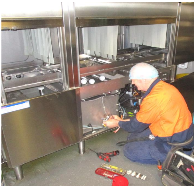
Pictured above: DES Electrical Contractor employee, Sandy Curran responding to a maintenance / repair call-out in the main servery, while at the same time adhering to the Home’s food safe protocol of wearing a hair net.
