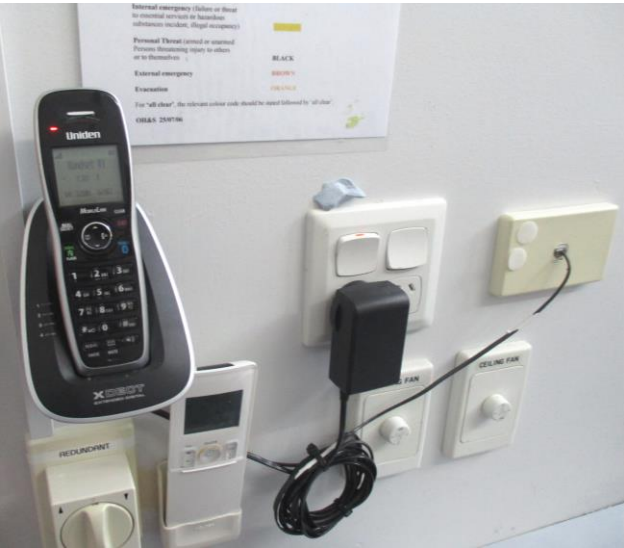
Pictured above: telephone cradle affixed to wall (LHS) in Banksia kitchenette to restrict easy access to non-staff personnel.
