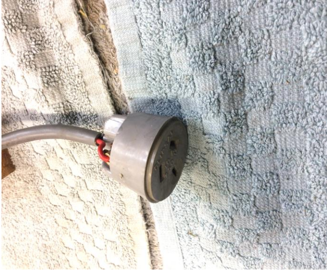
Pictured above: An electrical hazard that caused a staff incident which resulted in an electric shock.
